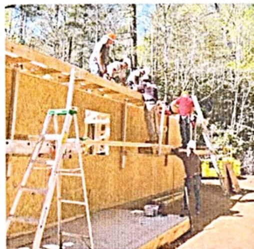
A new home being built by Brethren Disaster Ministries volunteers in Henderson County, N.C., for a Hurricane Helene survivor.
